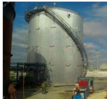
Industrial Storage Tanks
