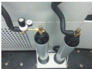
Fire Suppression System (CO2)
