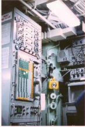
Ship-Board Communication Systems
